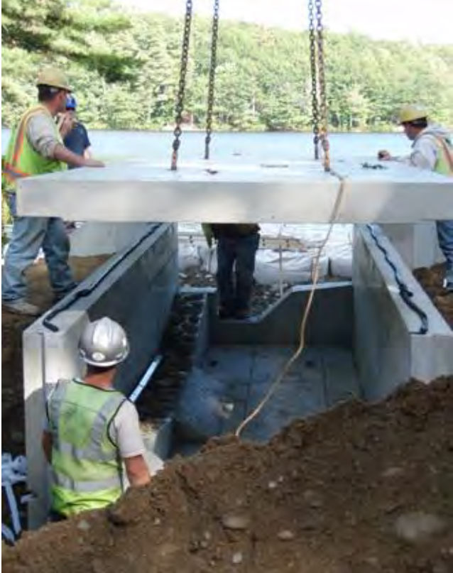
Installation of the new fish passage and removal of the existing outlet dam and fishway.
