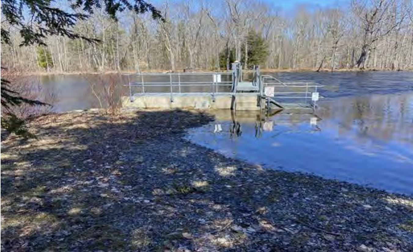
Newly installed fishway and overtopping of the dam during the river herring run.
