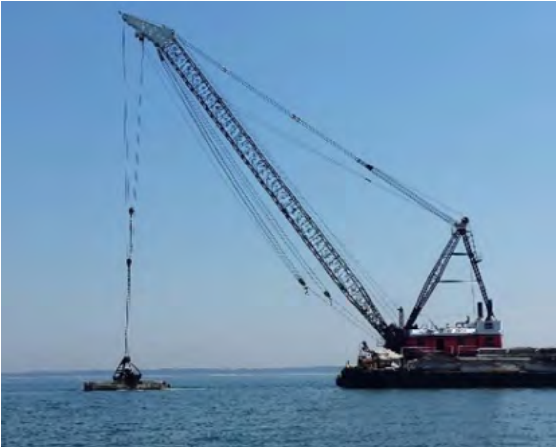
Figure 29. Deployment of Lesner Bridge material to the Cabbage Patch by McClean Contracting Company (2017). Photo credit: VMRC.
