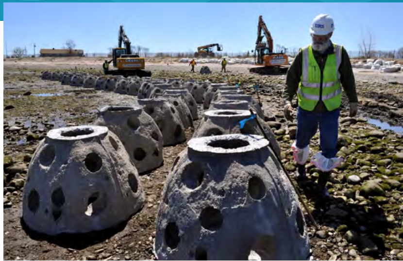
Figure 15. Precast concrete reef balls called Pallet Balls being deployed at the Stratford Point Living Shoreline in 2014. Photo credit: CT DEEP.
