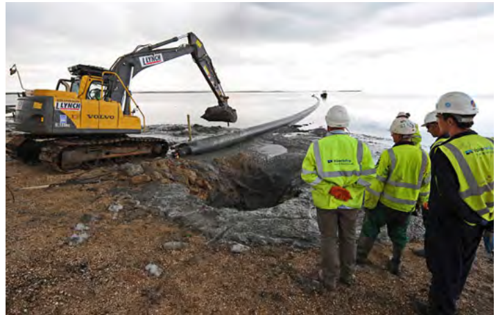
Offshore export cables
