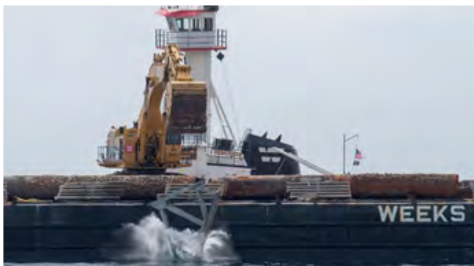
A piece of the Tappan Zee Bridge becomes part of a new patch reef. Photo credit: C. LaPorta, NYSDEC.
