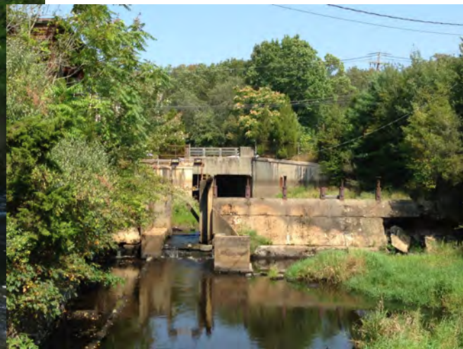
Cotton Gin Mill Dam, looking upstream (Source: Cathy Bozek, The Nature Conservancy)
