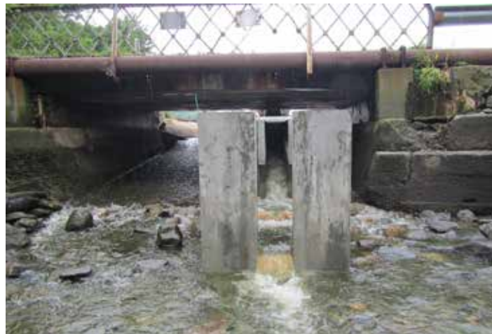
Beaver Lake Dam during construction. Photo credit: V. O'Neill Passage Seaward Side. Photo credit: S. Harold, TNC
