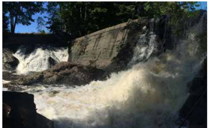
Gonic Sawmill Dam, Cocheco River, Rochester, NH. Photo Credit: K. Lucey, NHDES Coastal Program
