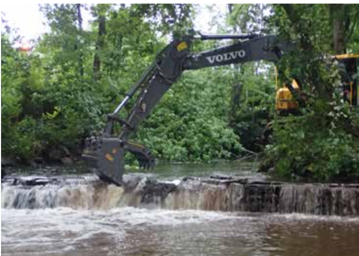
Even low dams like the Clark Bros Dam on the Quinnipiac River can block river herring runs. Photo credit: CTDEEP
