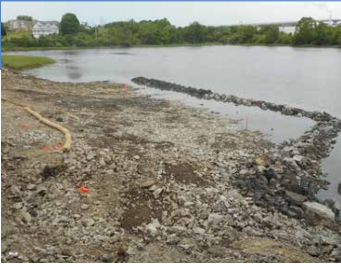
Cutts Cove Living Shoreline Project: construction of the rock sill associated with created intertidal salt marsh habitat. May 2017. Photo credit: NHDES, Coastal Program
