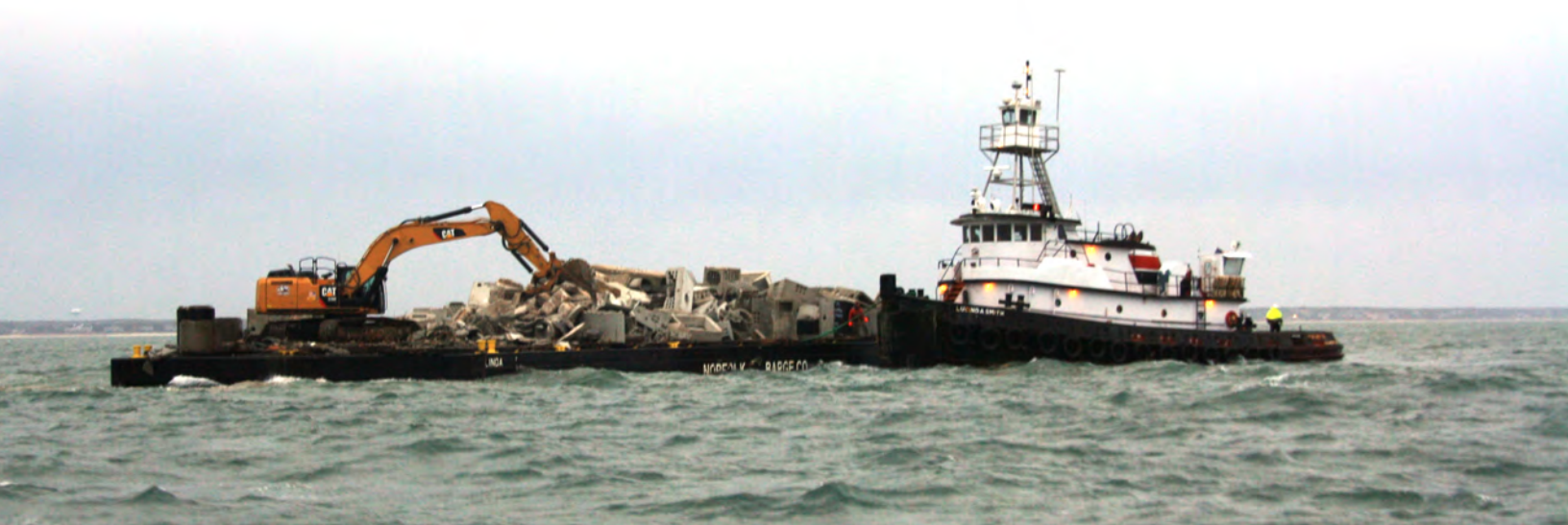
Figure 4. Deployment of materials to the Harwich Artificial Reef site. Photo credit: Mark Rousseau, MA DMF.
