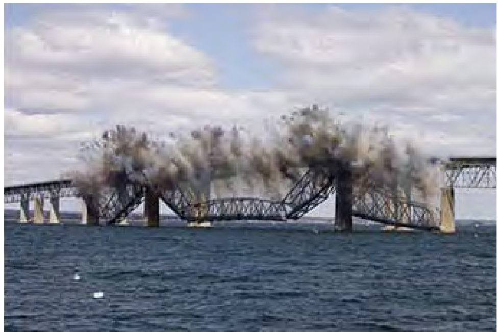
Figure 11. The through truss span of the Old Jamestown Bridge, just before it hits the water following the first controlled explosive demolition in 2006. Photo credit: RIDOT.
