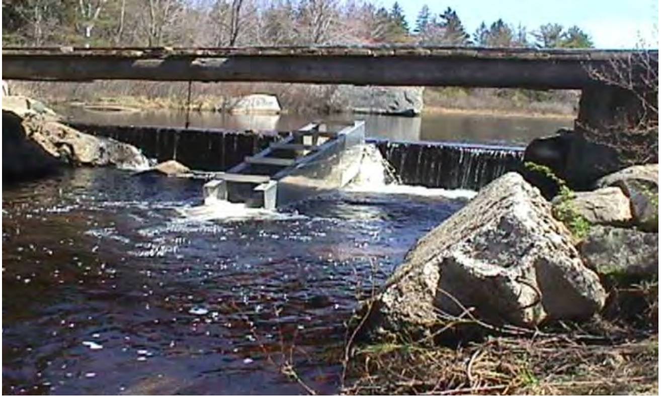
Old dam and fishway located at Wights Pond prior to installation of a nature-like fishway
