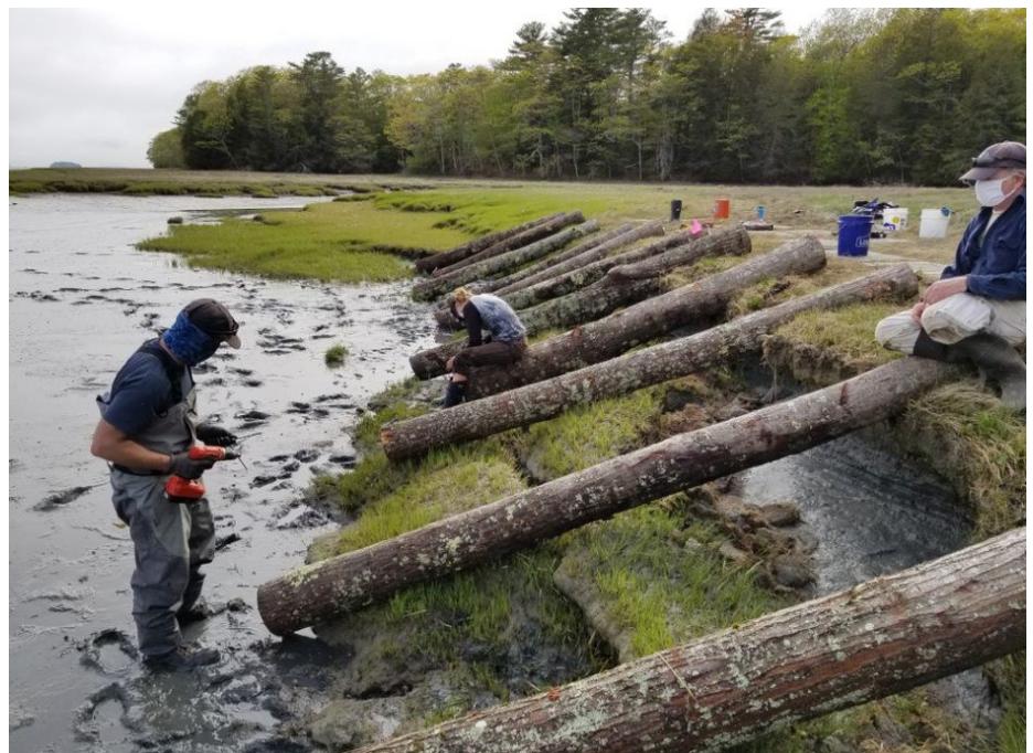
Living shoreline installation in Brunswick, ME. Image credit: P. Slovinsky, Maine Geological Survey.
